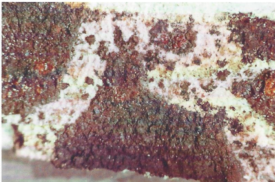
CORROSION PRODUCTS ON THE UNDERSIDE OF A BLISTER CAP
