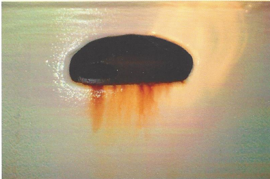
Inadequate stripe coating
